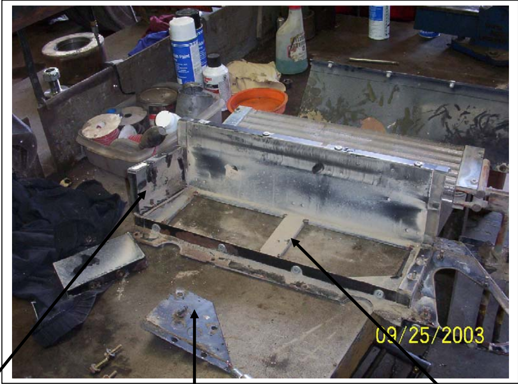
End cap flipped over so it cups out to accommodate the evaporator coil
