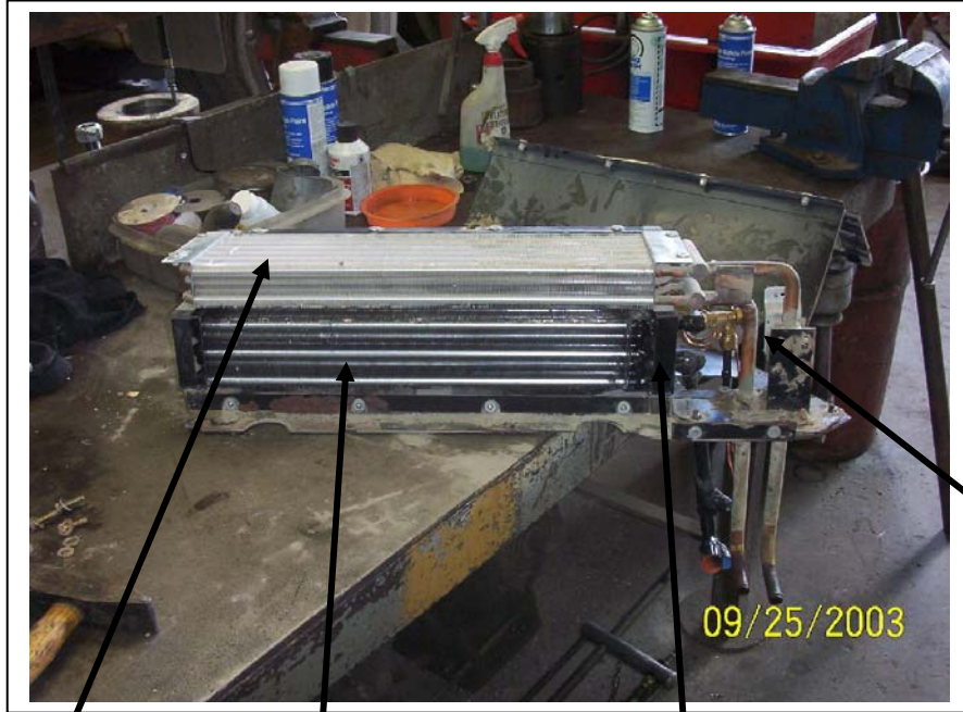
Heater coil back in place
